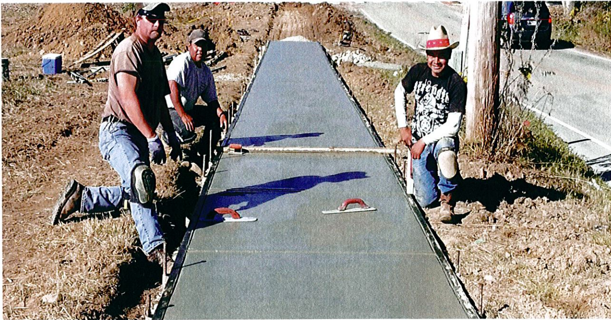
And the City of New Castle kept its promise to extend the Garner Street sidewalk to the WWT, making the trail even more accessible. Bike and foot traffic on the trail has surpassed expectations. Kudos to a healthy option for Henry County residents as well as visitors.
