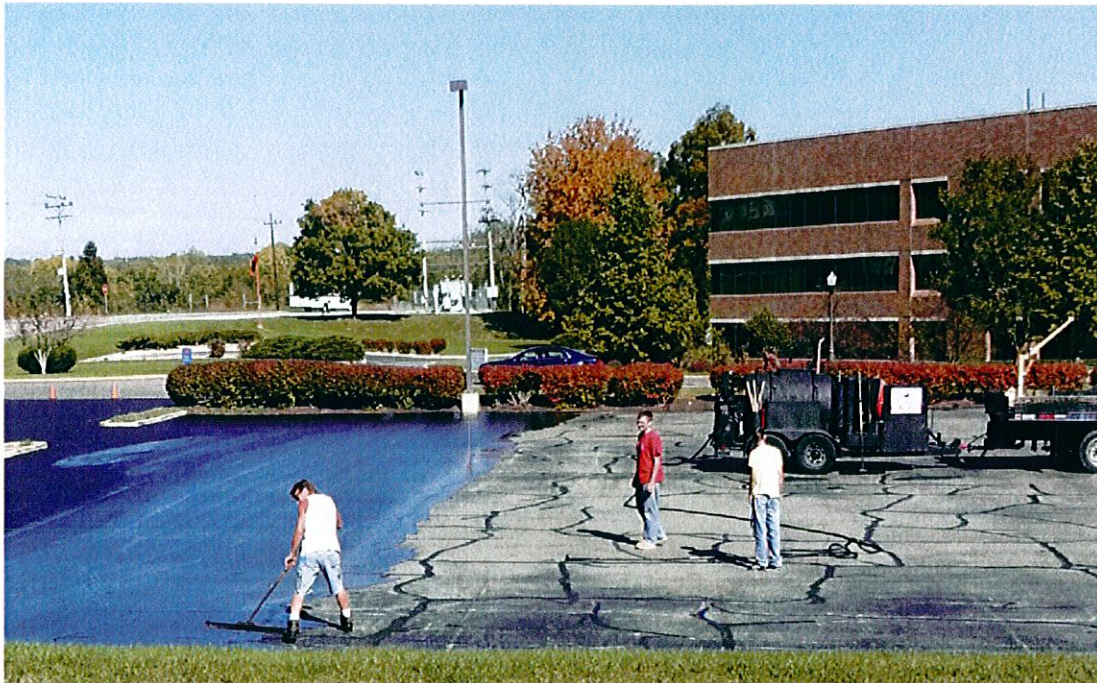
Maintaining excellence: Henry County Hospital re-seals its parking lot this October. (Lovely. Thank you!)
